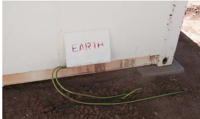
Figure 8: Earthing terminations on a steel relocatable magazine
