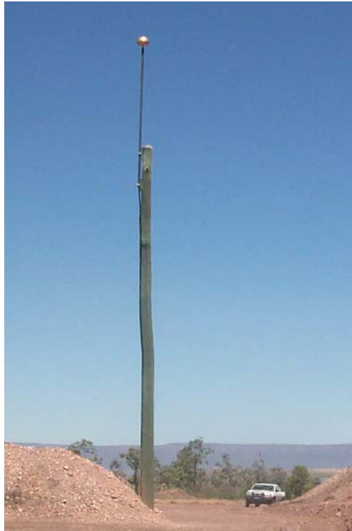
Figure 7: Vertical conductor used to protect relocatable steel magazines
