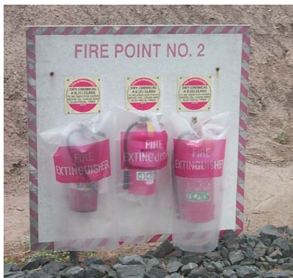
Figure 9: Fire fighting equipment clearly accessible inside the magazine perimeter
