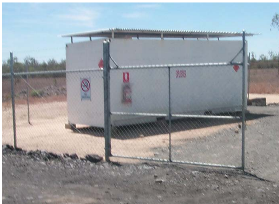
Figure 4: Magazine with chain and barbed wire fencing
